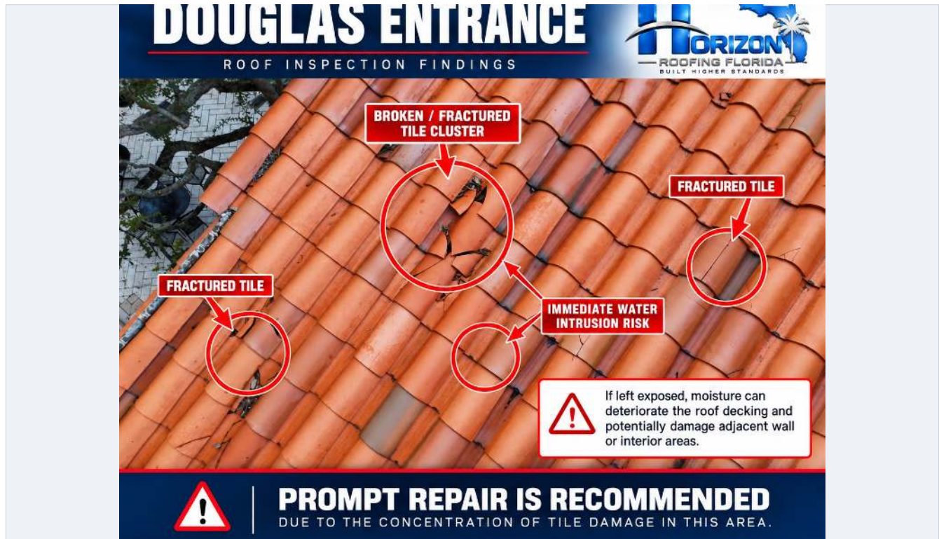
Douglas Entrance — fractured tile cluster; moisture intrusion risk
