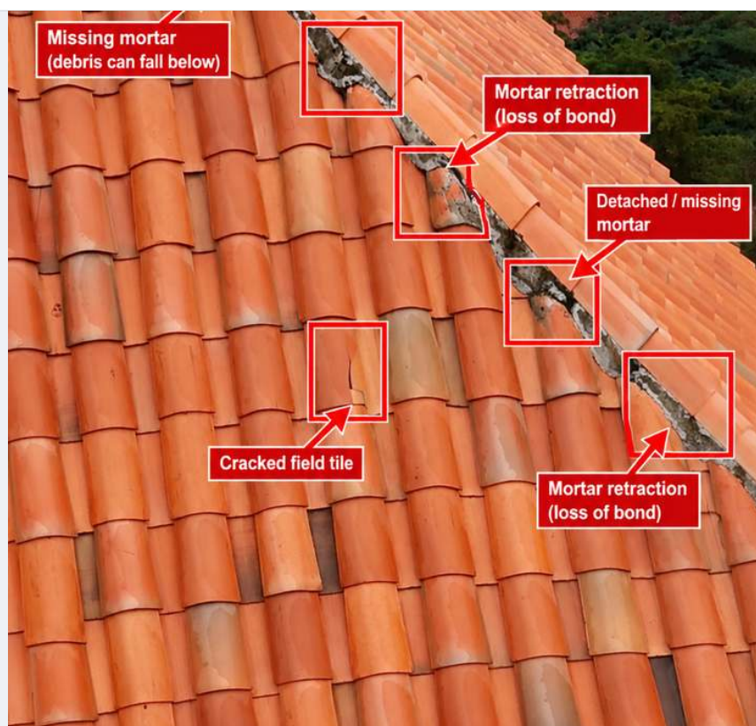
North Tower — cement/mortar cracking along bedding
