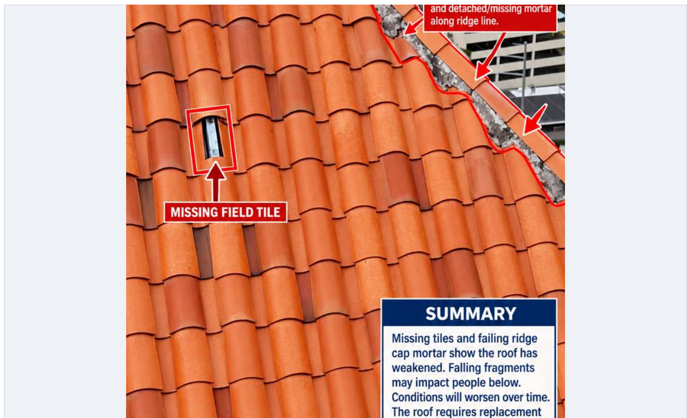
North Tower — ridge mortar brittle and deteriorating
