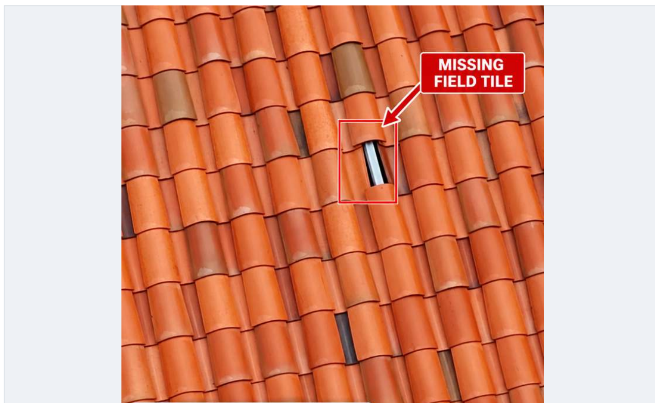
North Tower — missing field tiles; wind exposure at height
