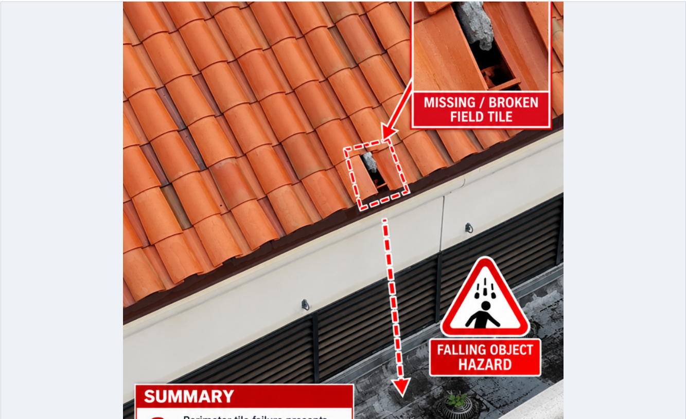
North Tower — broken and displaced clay tiles at elevation
