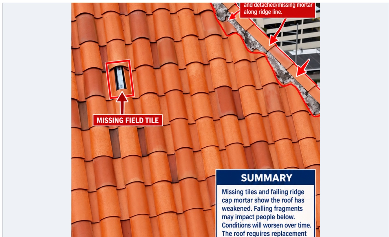
North Tower — ridge mortar brittle and deteriorating
