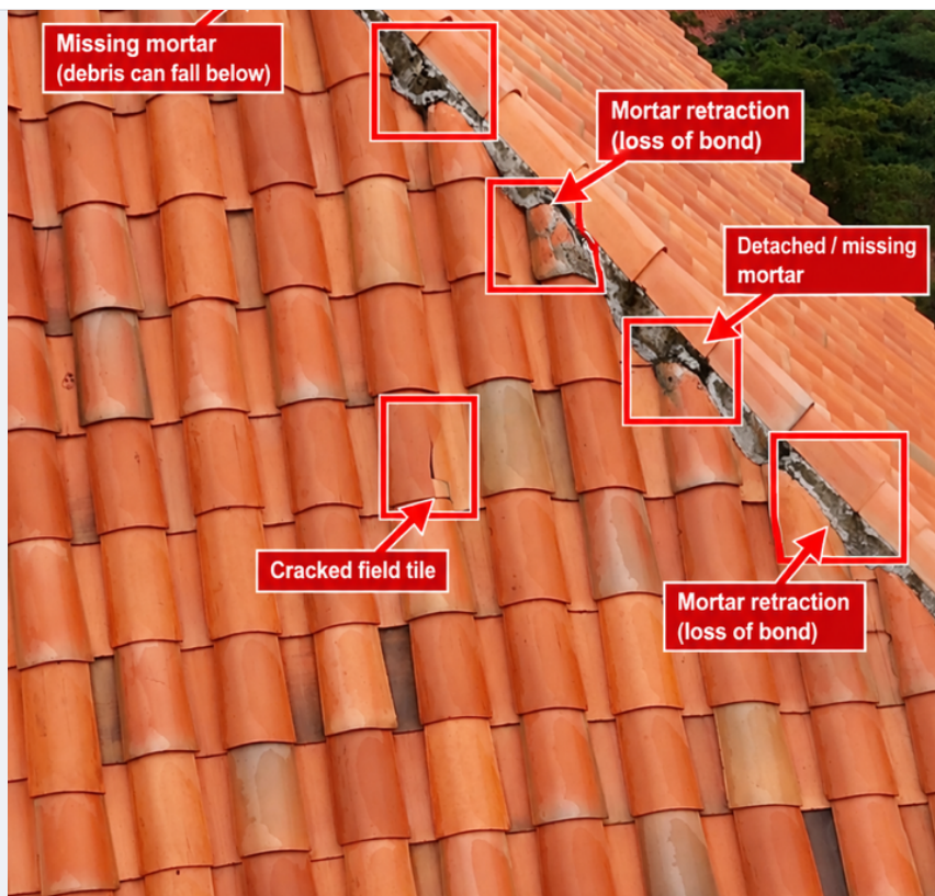
North Tower — cement/mortar cracking along bedding
